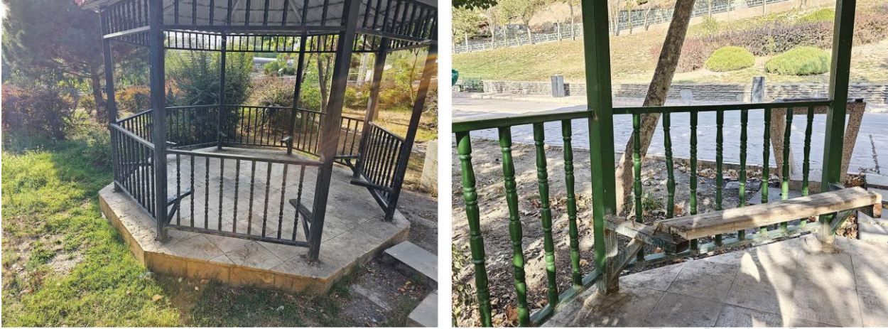
Figure 5. Inefficiency and severe damage to urban furniture in Javanmardan Park (Poorhasan Mehrzanjani, 2025)
